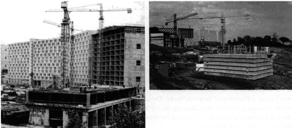
Figures 8 and 9. Construction process of the cellular structure, using the tunnel formwork technique. Sources: Mediathèque de Bayonne and Musée Basque et de l'Histoire de Bayonne (Photographs by Robert Hourgras).
